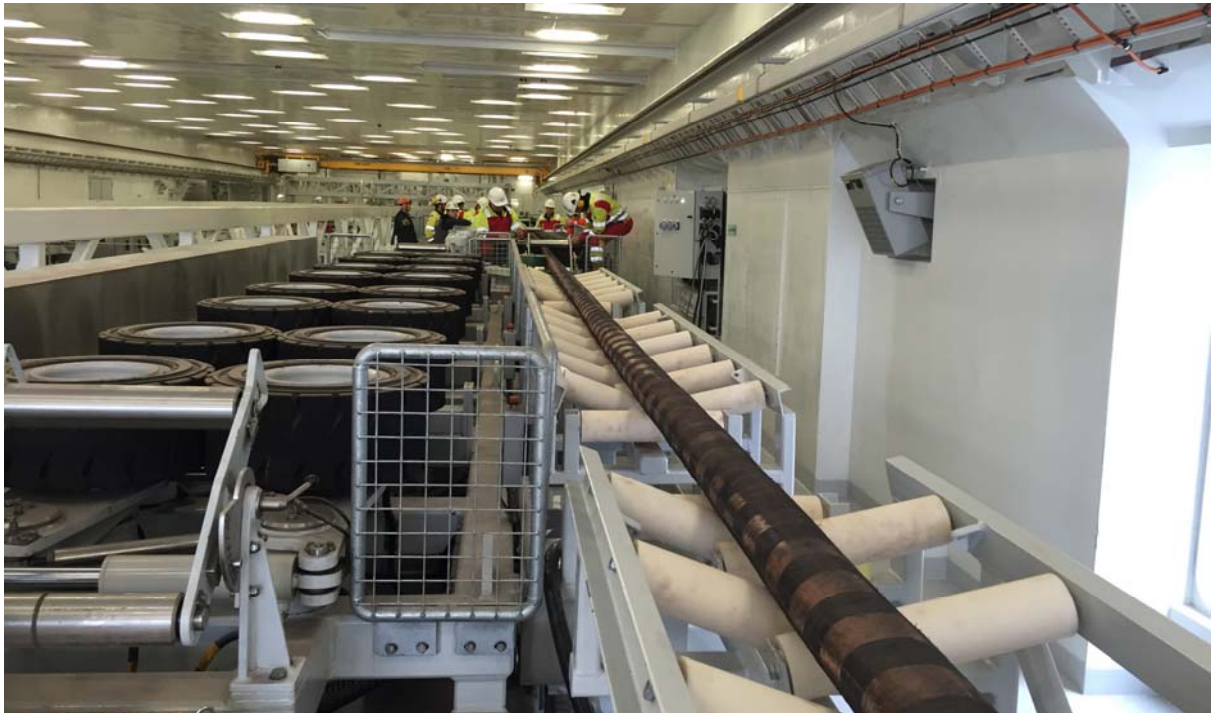
Arrangement on Cable Handling Deck
